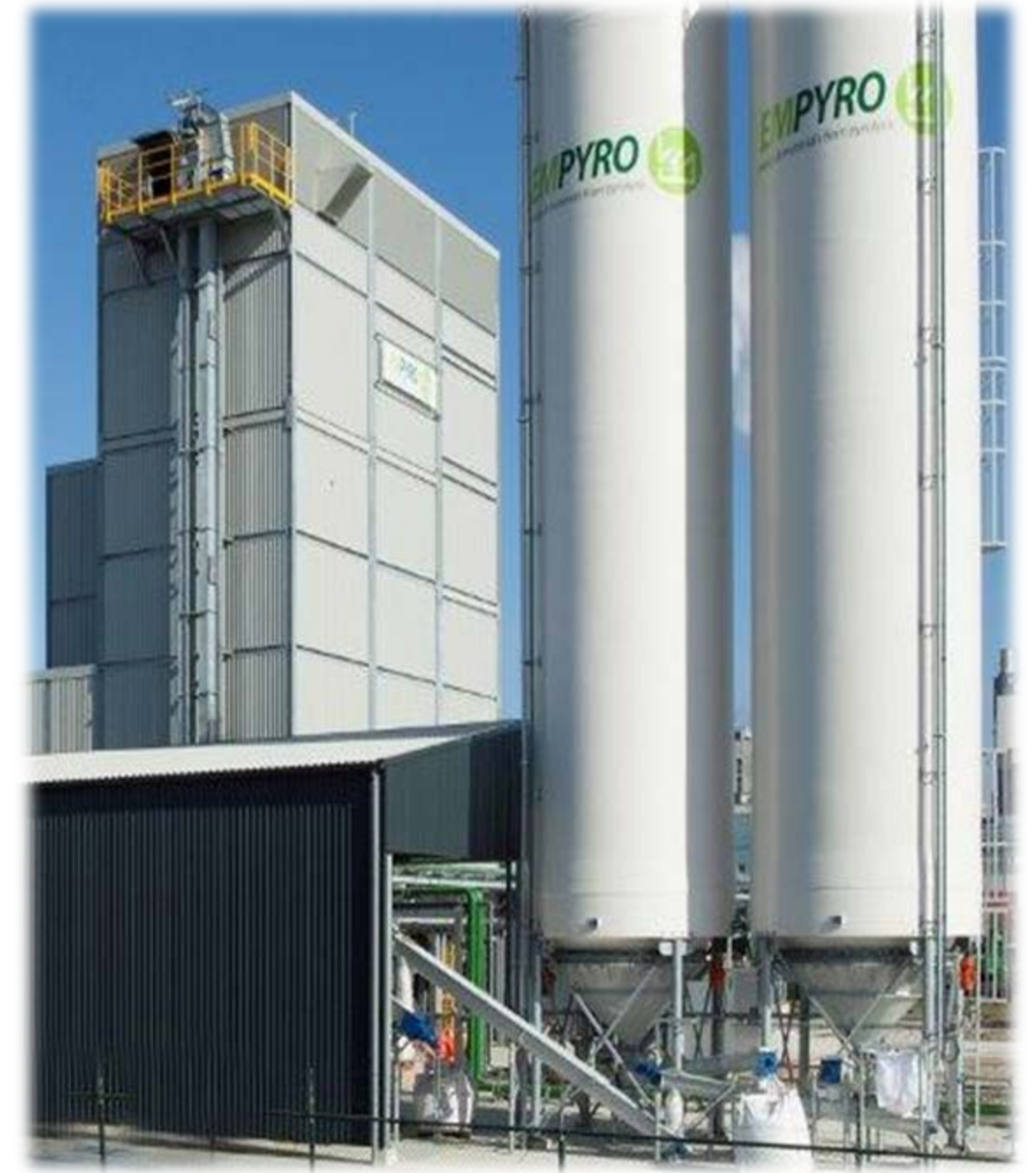
Empyro Hengelo Biorefinery (Netherlands)
